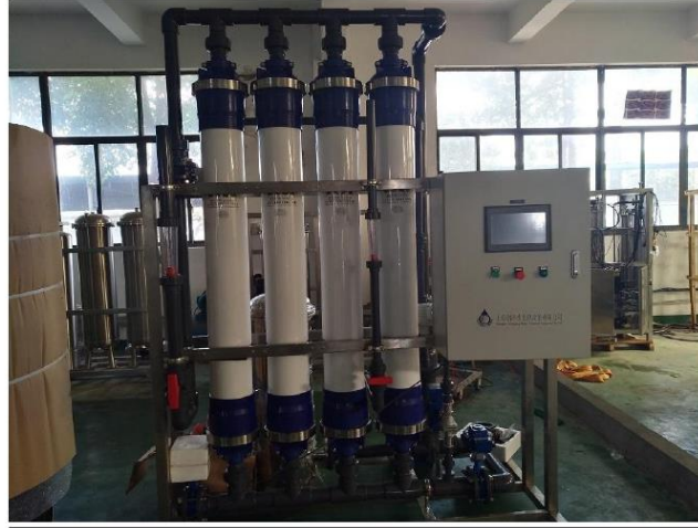
Ultra filtration System
